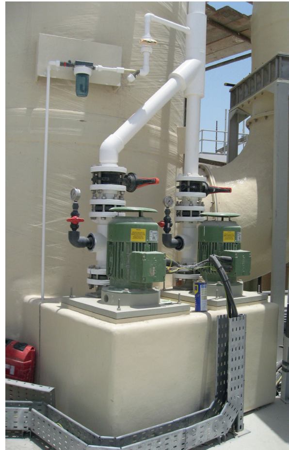
Immersible pumps on scrubbers
